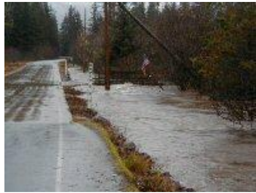
Montana Creek flooding.
